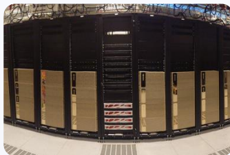
BERZELIUS SWEDEN DATA CENTER
